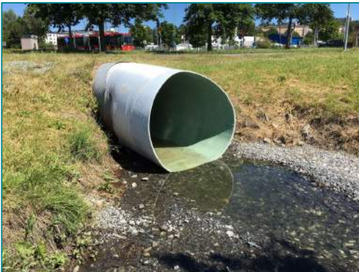
Successfully relined collapsing storm drain using DN 1400 underneath a park area in Järfälla, Stockholm.
