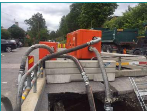
A complex pumping setup was required to enable successful installation of the liners.
