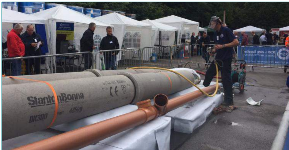
A demonstration installation of the Berolina-Liner in a DN300 pipe, at RSM's open day.
